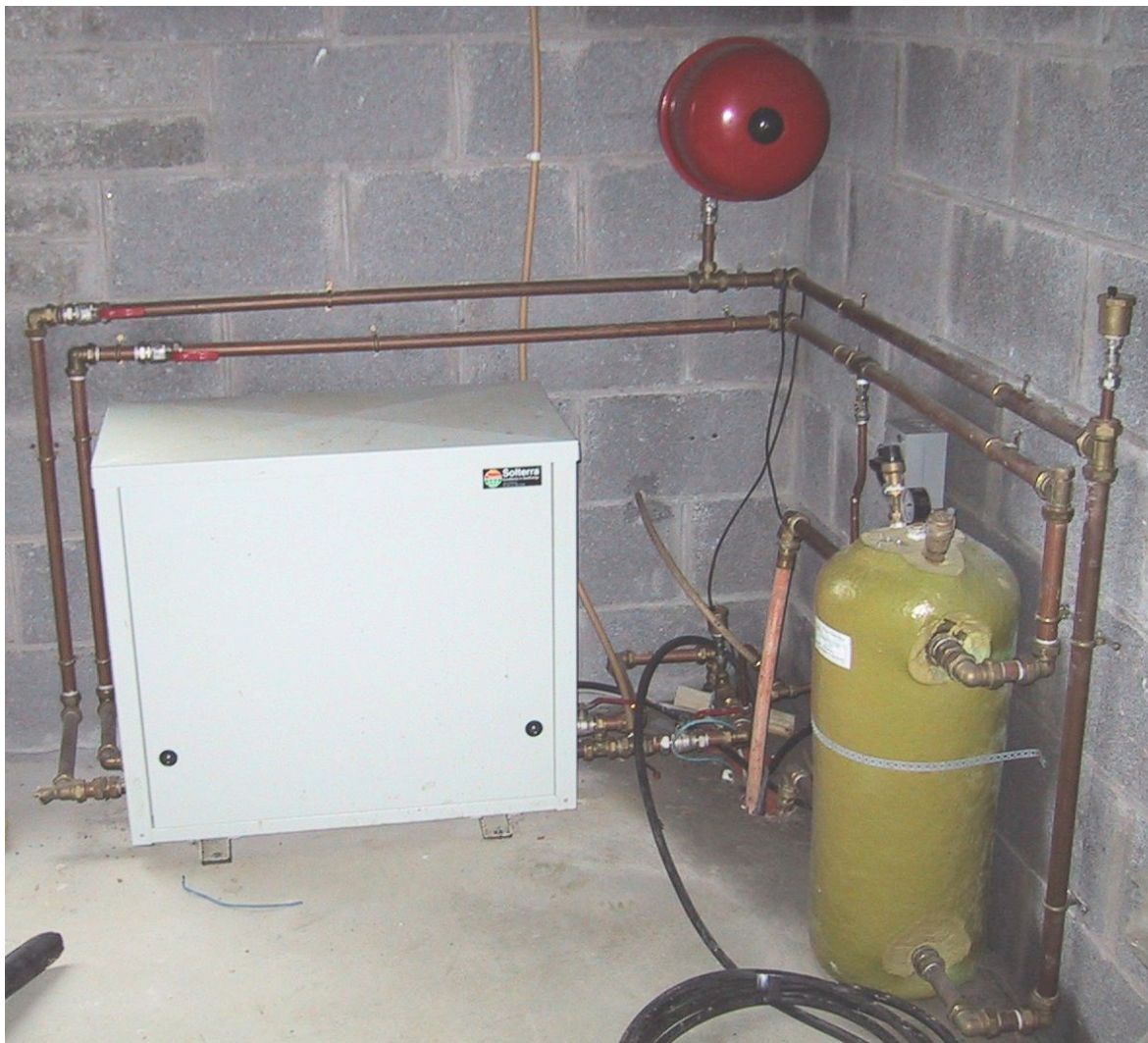
Image of a typical heatpump-in-situ
