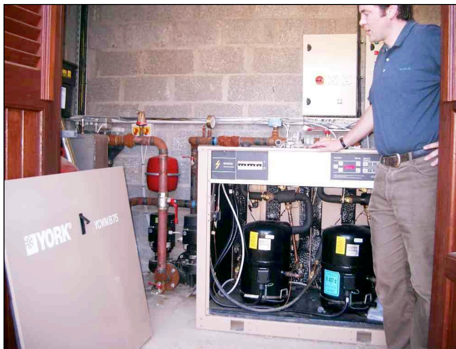
A large heat pump room
